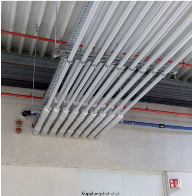
Specially secured wall penetrations for material lines in fire protection walls (Source: motan)
